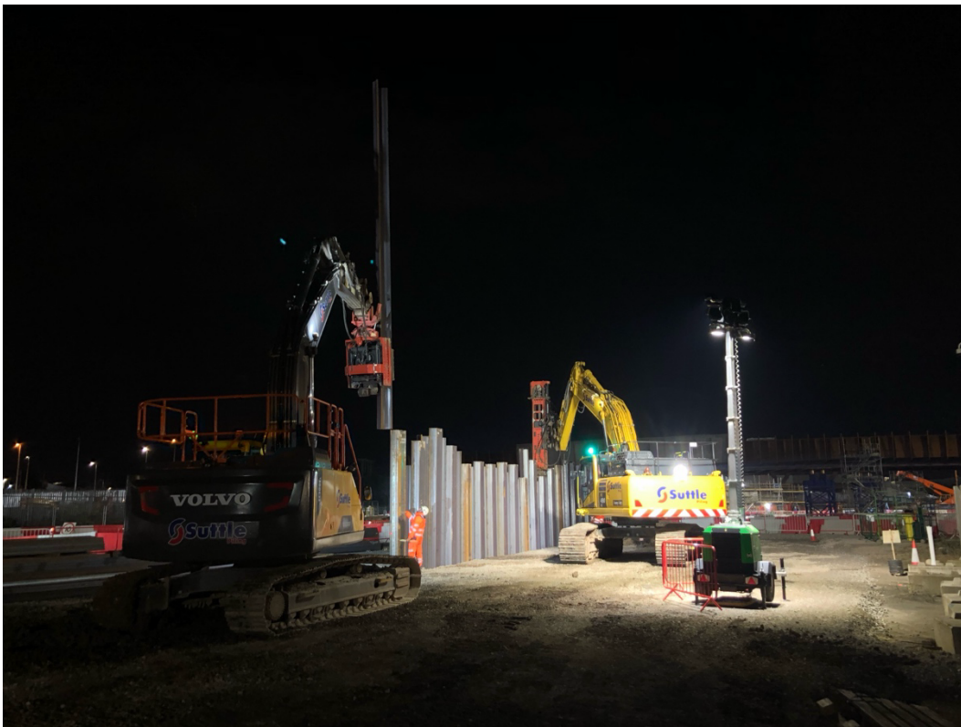
Figure 2: Our Volvo EC330 and Komatsu PC490 during a nightshift completing some sheet piling.
